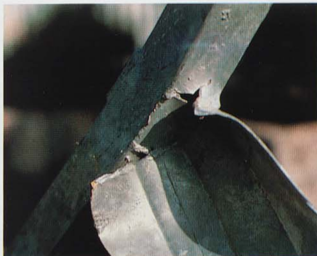
Fig. 1: Explosion Damage due to improper venting.
