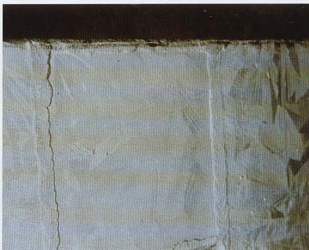
Fig. 3: Thick galvanized coating on weld due to high silicon content.
