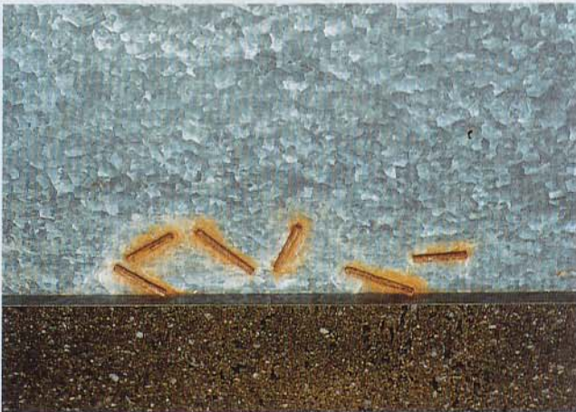
Fig. 4: The remains of welding rods can be the cause of "phantom rust".
